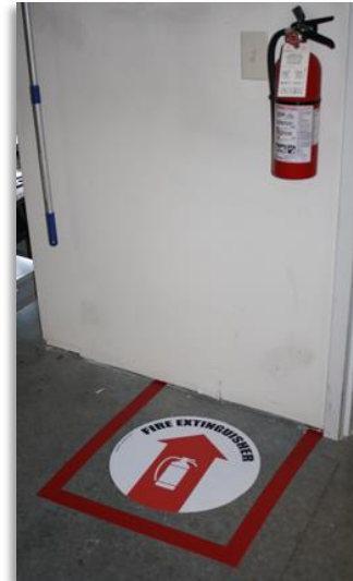
Line marked fire extinguisher location
