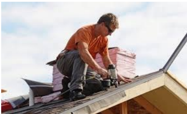
Person on roof at home without handrails or harness
