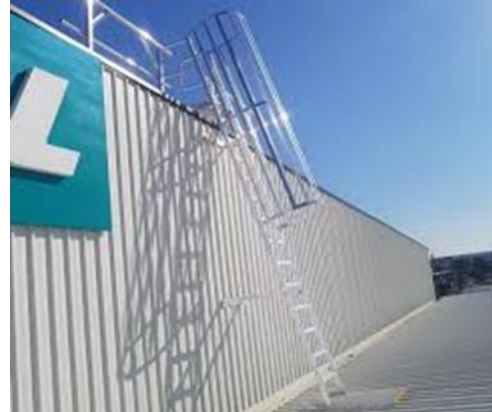
Safe roof access system
