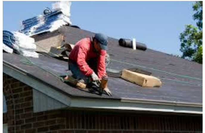
Sample scene showing a worker near an unprotected edge
